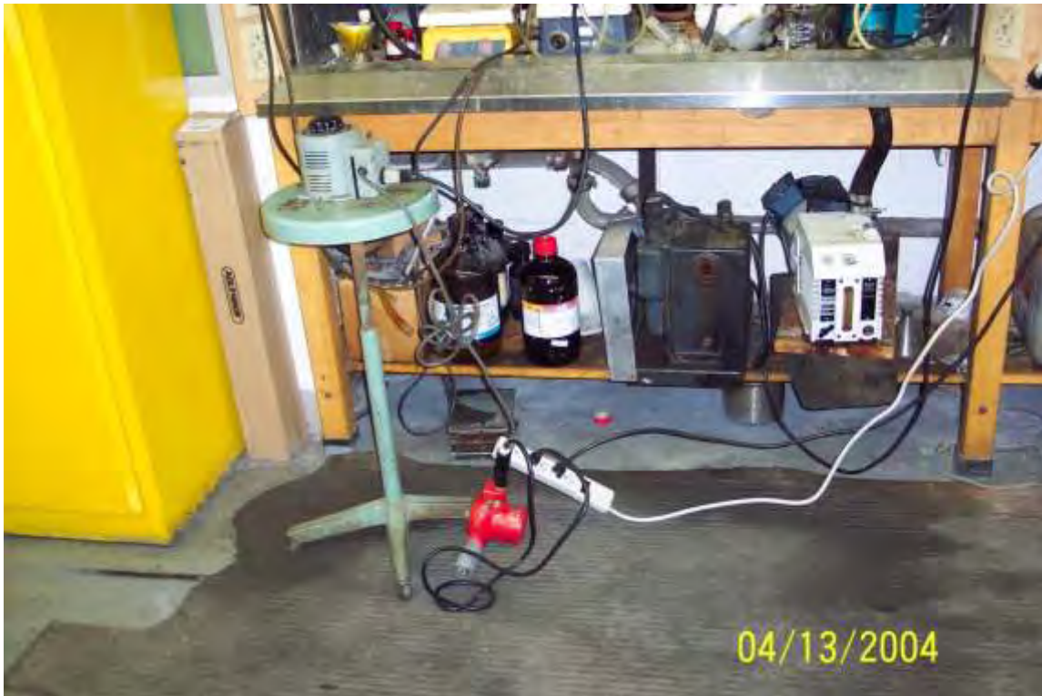
Fig 5.1.1.1: Example of a Potential Accident Area
